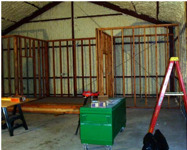
Insulation has been blown in and the framing is in for the bathroom and studio areas.
