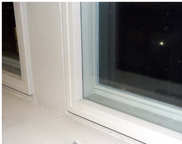
The inside window in front of the outside window. This piece of plate glass reduced noise from outside by greater than 60dB.
