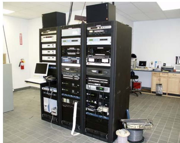
Equipment racks at the transmitter site.
