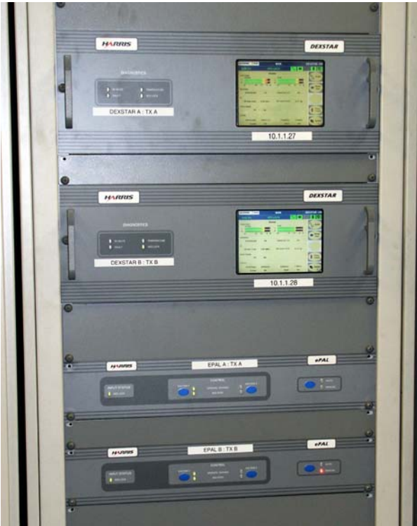
The HD rack sits between the transmitters. Each transmitter has its own HD exciter.
