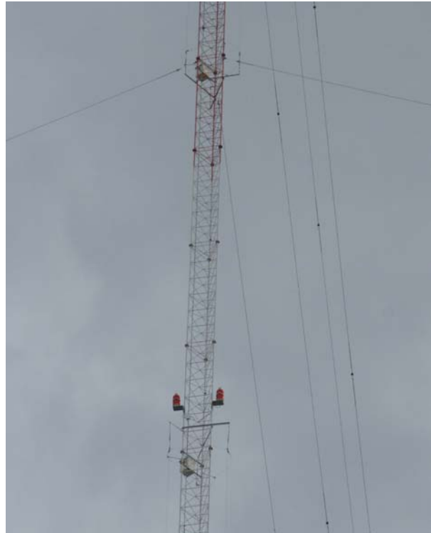
The detuning skirts can be seen, one below the center beacons, one just above where the orange section starts above the beacons. You can also see the capacitor boxes.
