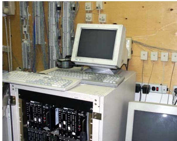
The Mitel PBX in its new home, the utility room near the Producer/Talent end of the floor.
