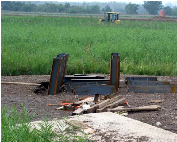
A guy anchor location. Note the angled piles on the left, toward the direction of guy wire pull.
