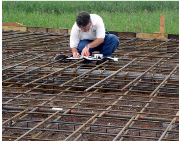
Paul Mucci of Civil Engineering firm Aerial Spectrum checks foundation rebar placement against the drawings before the transmitter building foundation is poured.
