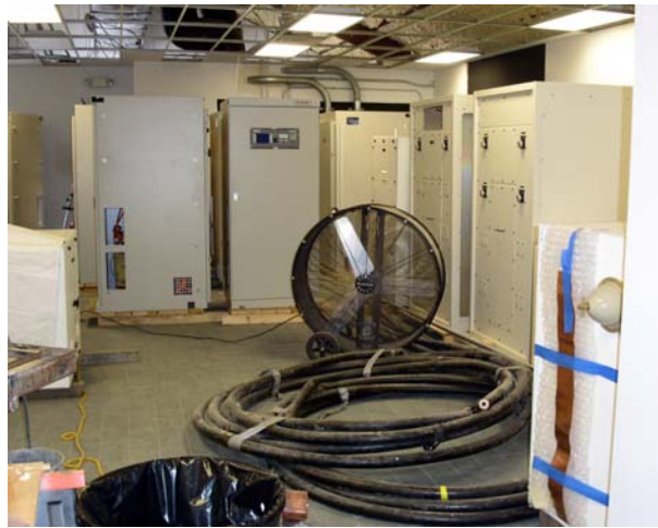
The transmitters and phasor have just been delivered to the WOR site.
