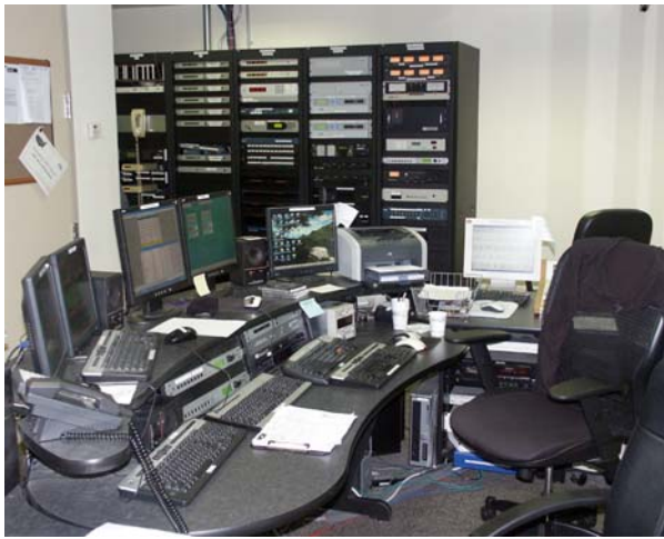
The WOR Master Control Room at 111 Broadway.
