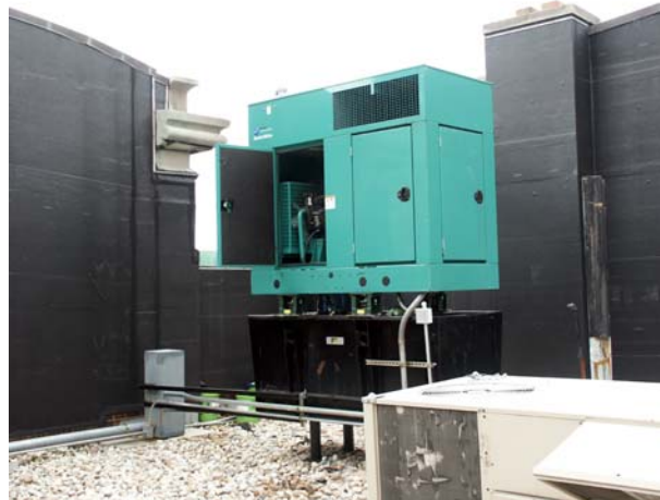
The generator sits in the south-west corner of the roof, hidden from street view by the facade. Ironically, the generator is almost the same color as the penthouse.
