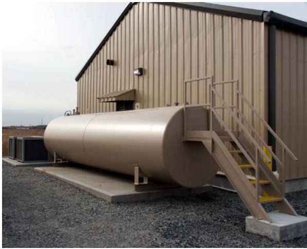
The 4,000 gallon diesel tank in place.
