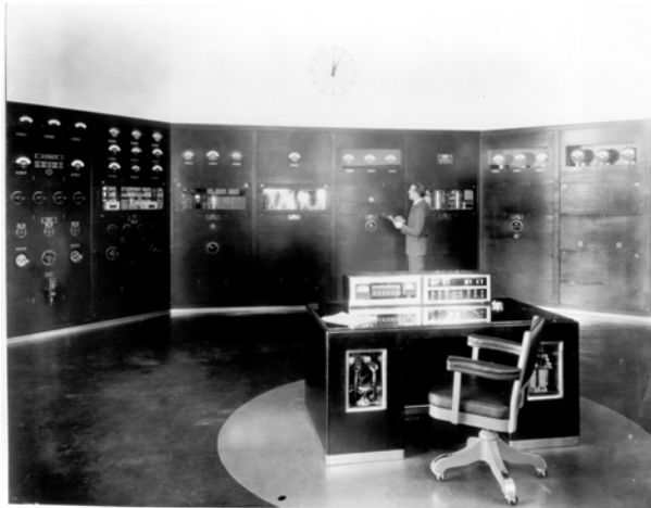
The Western Electric 50KW transmitter at the Carteret, New Jersey transmitter site. The Engineer in the photo is unidentified.
