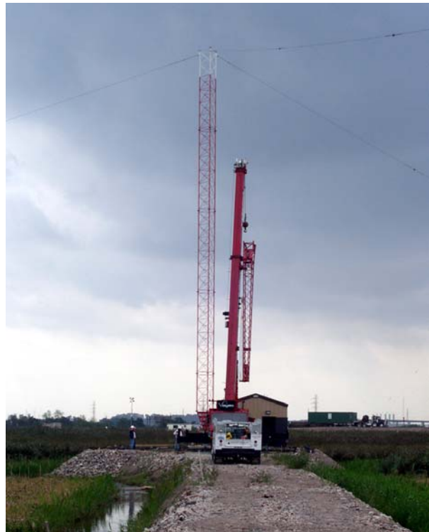
The first one hundred feet of tower 2 stands as the crane is lowered.
